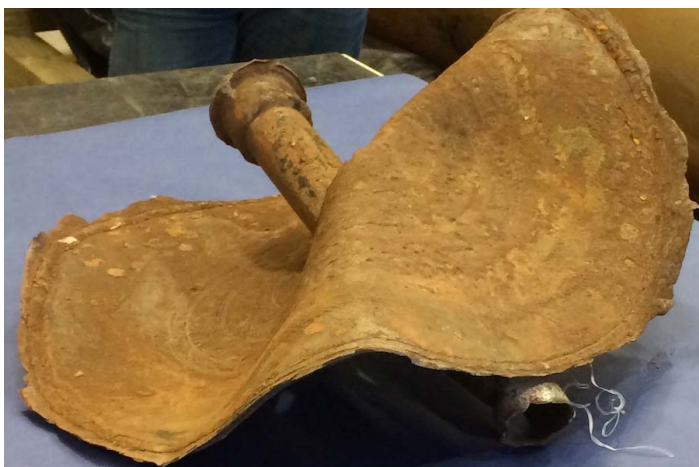
Figure 8. Close-up of bottom tank circle and portion of bottom piping showing weld seam and, outside of the seam, the thinned original bottom head “ring” material
