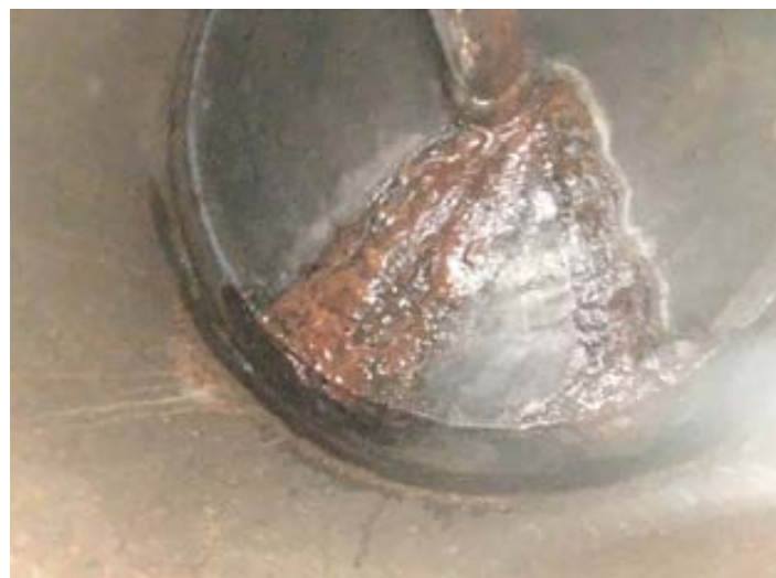
Figure 5. Photograph of SCR bottom head leak, taken March 31, 2017
